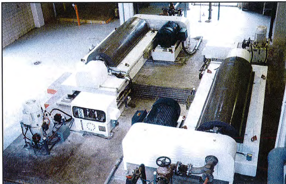
CENTRIFUGES are used to "spin dry" the BIOSOLIDS .
