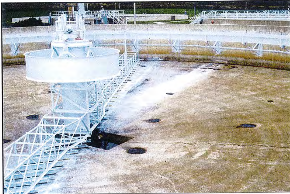
An empty PRIMARY CLARIFIER .
