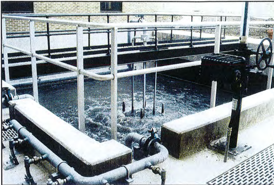
AERATED GRIT CHAMBERS remove sand and gravel.
