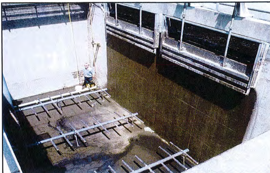
An empty aeration tank with FINE BUBBLE DIFFUSERS .
