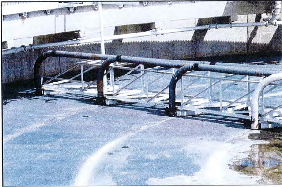
Empty secondary clarifier with "bug vacuum cleaner" .
