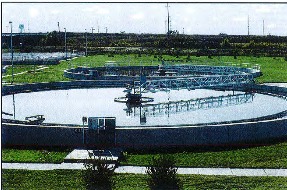
PRIMARY CLARIFIERS settle out some of the organic matter.
