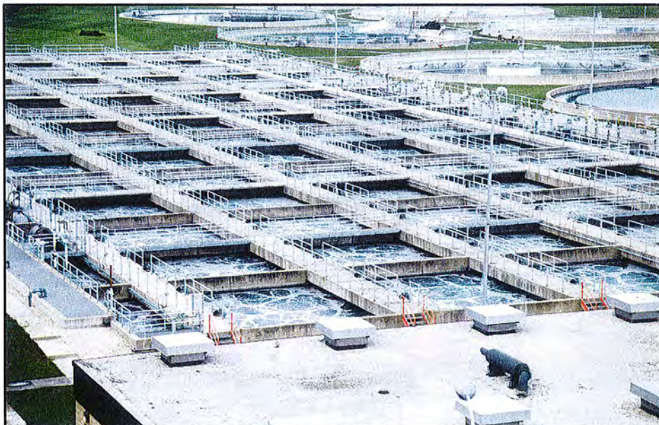
AERATION TANKS , where most of the cleaning is done.
