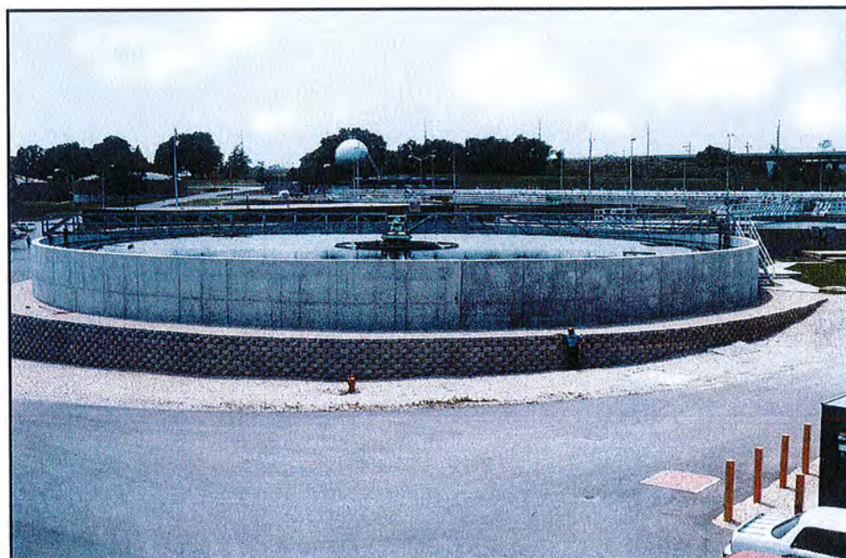
SECONDARY CLARIFIERS are used to remove "the bugs".
